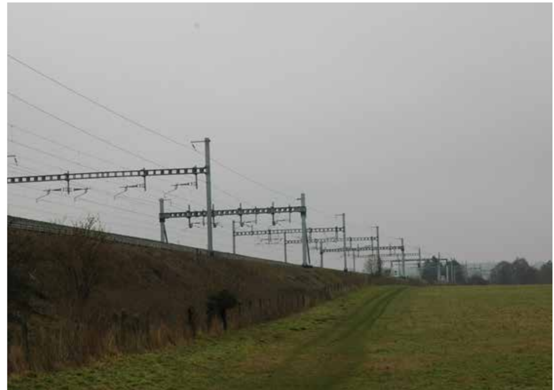
Gantry OLE structures
